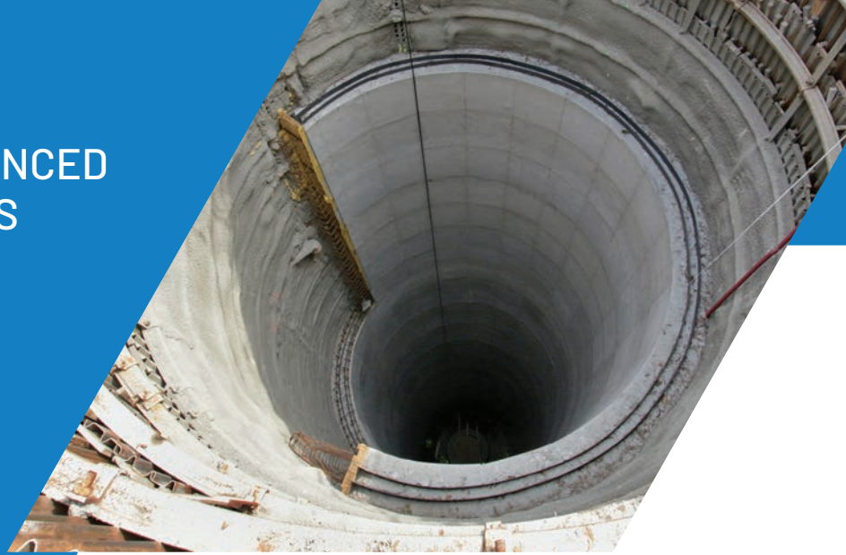
Prague Sewer Tunnels, Ďáblice, Prague, Czech Republic
