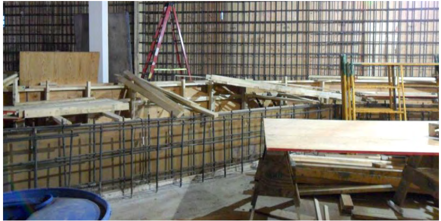
Fig 8 -- Engineers determined that the aquarium tanks could be built in the Powerhouse lower level as long as they were self-supporting and did not require the building walls for support. Much of the original character of the 1892 building was preserved.
