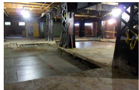
Fig 7 -- The basement of the Powerhouse required extensive renovation and reconstruction to accommodate the unique needs of the Greater Cleveland Aquarium. Engineers determined that the timber piling foundation could support the weight of the concrete and acrylic tanks, as well as the nearly 500,000 gallons of water the tanks collectively hold.
