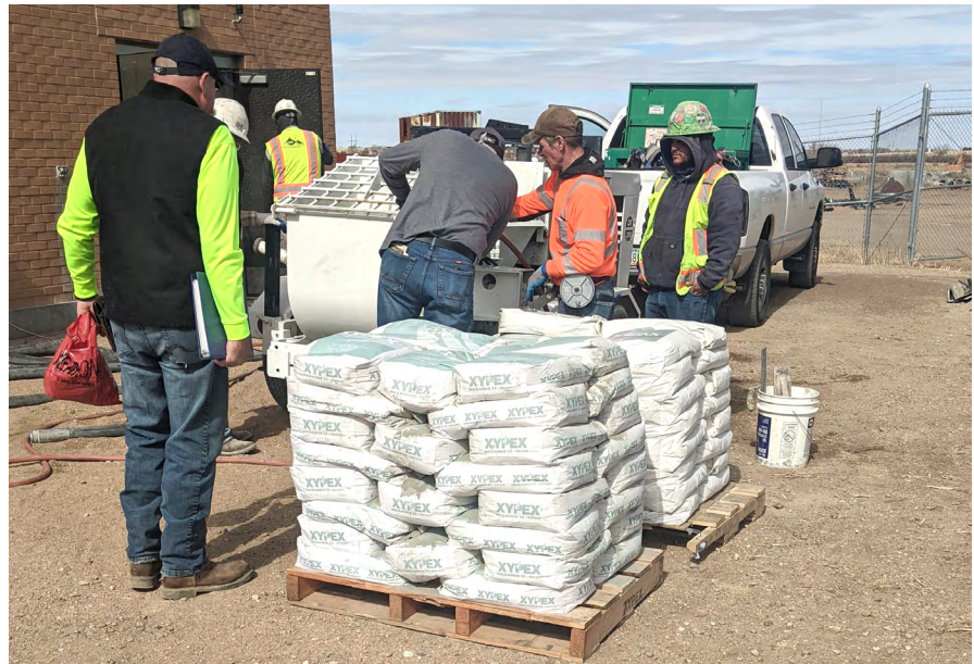
Fig 7 -- Colorado-based Advanced Shotcrete mixes Xypex Megamix II with Bio-San and pumps it nearly 30 feet below grade to spray apply it to the inner surfaces of the Lamar, Colorado, headworks facility.
