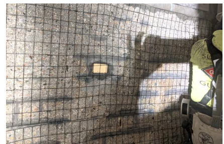
Fig 8 -- After hydrodemolition has removed all loose concrete and other debris from the wet well walls, exposed rebar is coated and sacrificial anodes are attached prior to the application of Xypex Megamix II with Bio-San.
