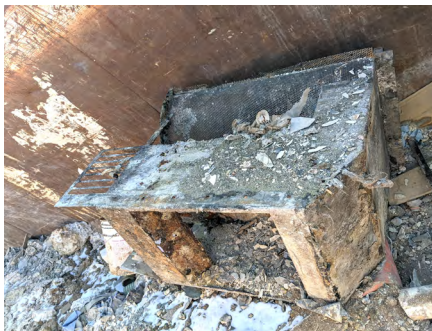
Fig 6 -- Even stainless steel was no match for the extreme corrosive effect of hydrogen sulfide gas and the resulting microbial induced corrosion (MIC). Here, the remains of a stainless steel filter are shown.
