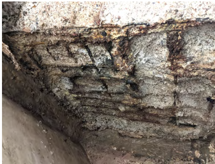
Fig 5 -- Concrete structures were deeply damaged by biogenic corrosion, resulting in concrete spalling and exposed reinforcing steel. An epoxy coating was applied within a few years after the structure was built, but failed quickly.
