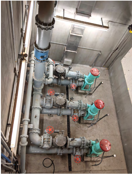
Fig 2 -- Half of the Lamar headworks is used as a pumping station to move wastewater out to a lagoon system just east of the facility. The other half is a wet well where influent is filtered.
