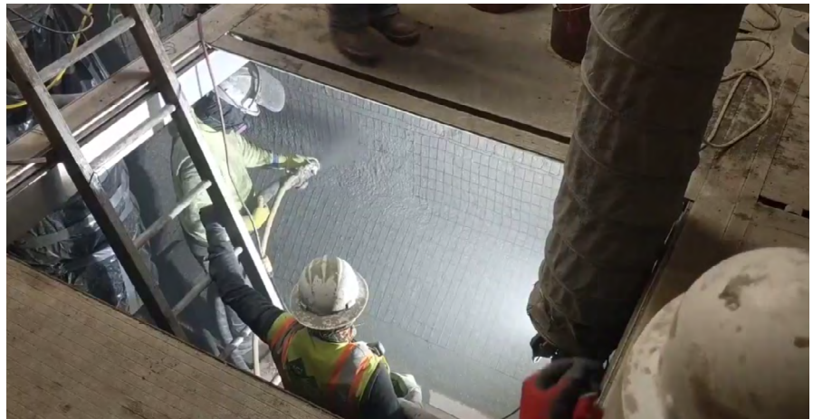
Fig 9 -- Applicator Advanced Shotcrete spay applies Xypex Megamix II with Bio-San during a restoration project at the Lamar, Colorado, headworks facility. In less than 10 years of service, extreme corrosion from excessive hydrogen sulfide gas caused rapid concrete spalling and metal corrosion.
